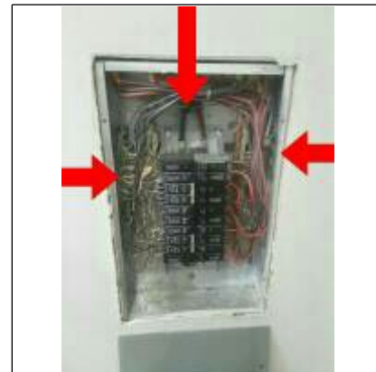
All neutral and ground are isolated on the bus bar.
