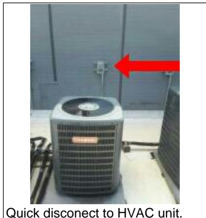
Quick disconnect to HVAC unit.
