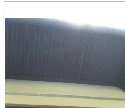
Metal grade under balcony.
