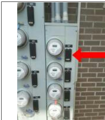
Quick disconect to meter box.
