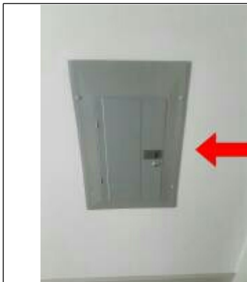
Subject panel appears to be satisfactory behide master bedroom door.
