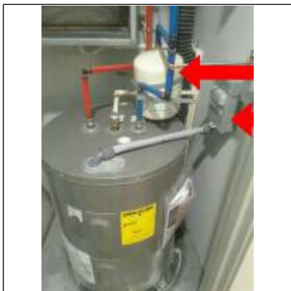
Water pressure system. Quick disconnect to water heater.
