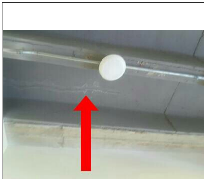
Settling crack. Also possible leak due to the efflorescence on the surfaces.
