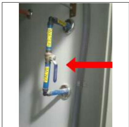
Main shut off for unit.
